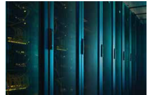
Piller returned to the hyperscale data centre sector with its M+ Series Battery UPS at Data Centre World Frankfurt in May.
